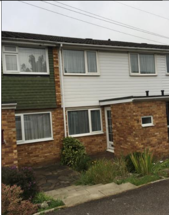
Negative thresholds along Napier Drive – showing steps down to houses, presenting areas of ponding/vulnerability to houses
