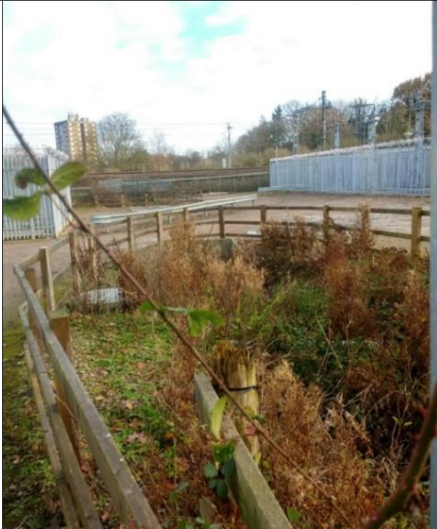
Section of open channel upstream of Blair Close, located within the land owned by Rail Electrification Alliance.
