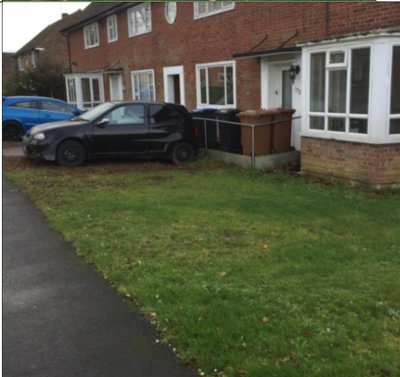
Image of property on Marley Road that has experienced flooding in the past on a number of occasions. Low thresholds towards entrance to property.
